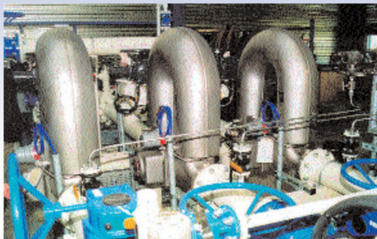
A crude oil custody transfer unit based on mass flowmeters ELITE CMF400
