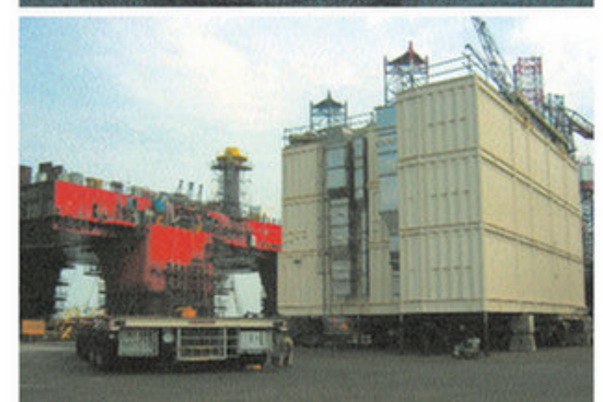
During loading at Singapore a giant barge crane - Asian Hercules, with a lifting capacity of 3200 tons - was used.
