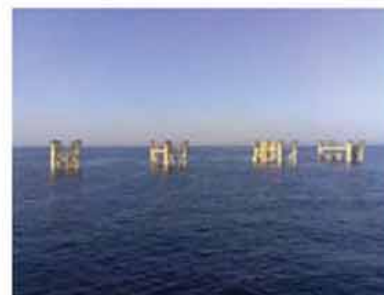
DUQ and PCWU jackets in Position and Docked onto the Pin Piles.
